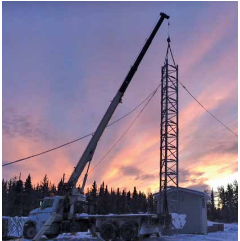
Cell tower in Black Lake. Photo courtesy of SaskTel.
